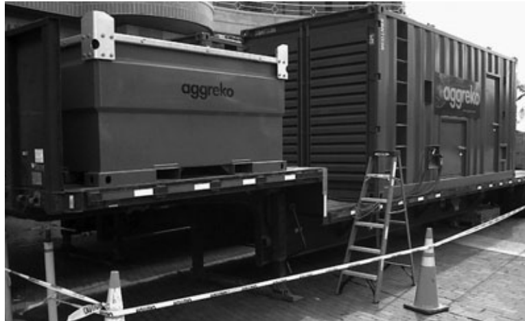
Washington Harbour cleanup generators
